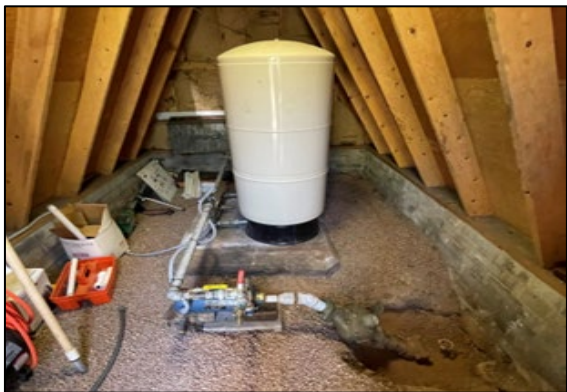
VG2 Pump & Bladder Tank
