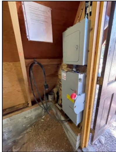
Electrical Controls at VG2
