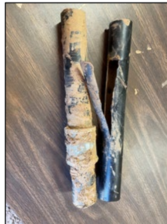
ABS plastic pipe likely broken under the weight of vehicle due to inadequate ground cover
