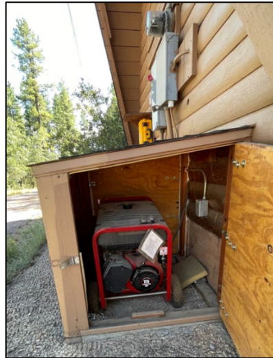
Mobile Emergency Generator stored at VG1
