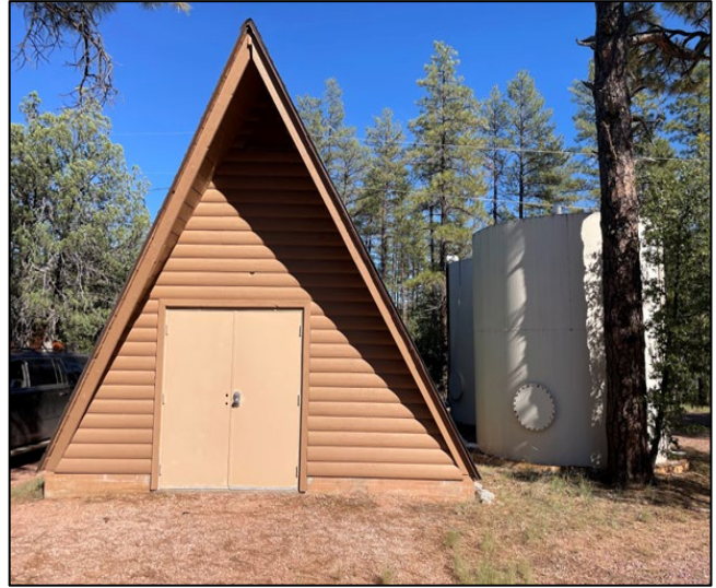
VG1 Facility (Booster pump, chlorine system and pressure tank)
