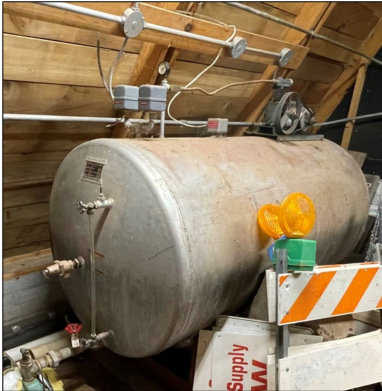
HP Tank at VG1 Pump House
