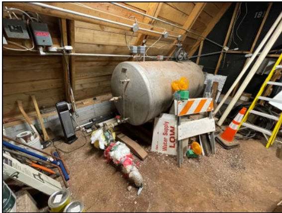
VG1 Pump & HP Tank
