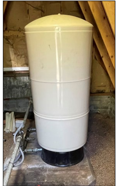
Bladder Tank at VG2 Pump House
